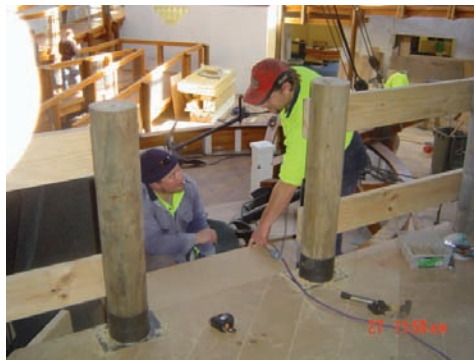
Luke and Mick - Project Hahn - working on the steps to the Norfolk-providing safe limited access.
