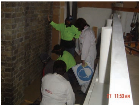
Back walkways get the finishing touches –Judy & Rosemary plus some of Project Hahn.
